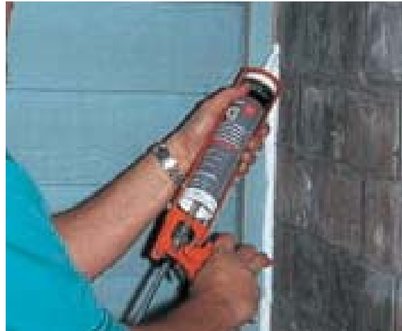
Caulk upward, pushing a bead of paintable caulk in front of the nozzle as you work.
