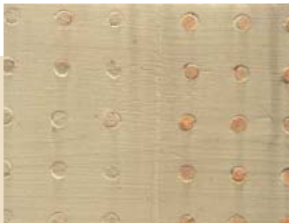
Rusted nail heads (courtesy Behr/Rohm and Haas).
